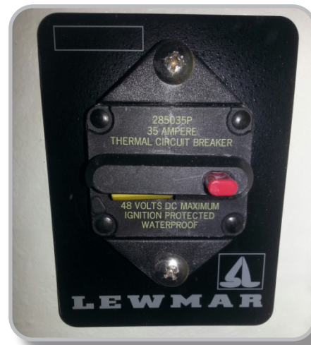
The windlass breaker is located in the head/console compartment.
