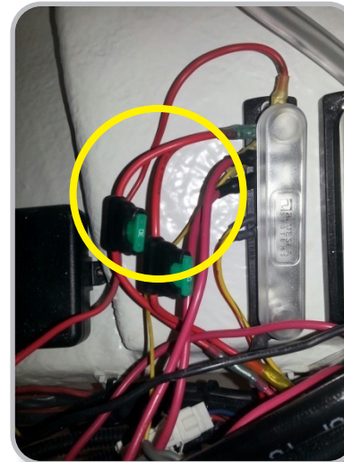
The fuses for both the marine head and the waste tank are located behind the dash in the first panel coming off the bus bar, pictured to the left.
