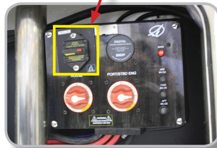
The windlass breaker is mounted on the VSR Battery Switch Panel in the Bilge.
