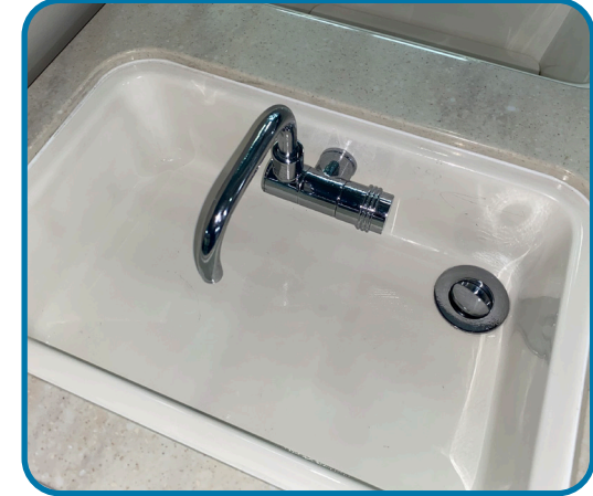
Galley - Freshwater Sink with Pullout Shower
