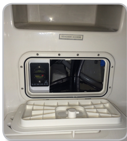
The windlass breaker is located in the bilge hatch below the walk-thru transom door.
